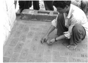
Cleaning the frog of the brick from wet sand for better binding
