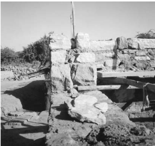
Bad example, stone wall construction without bond stones
