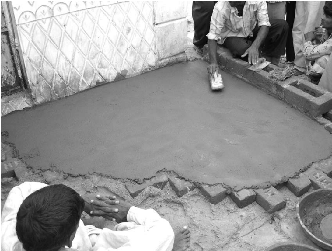
Floor construction section, levelling sand, brick layer, cement cover and finishing work
