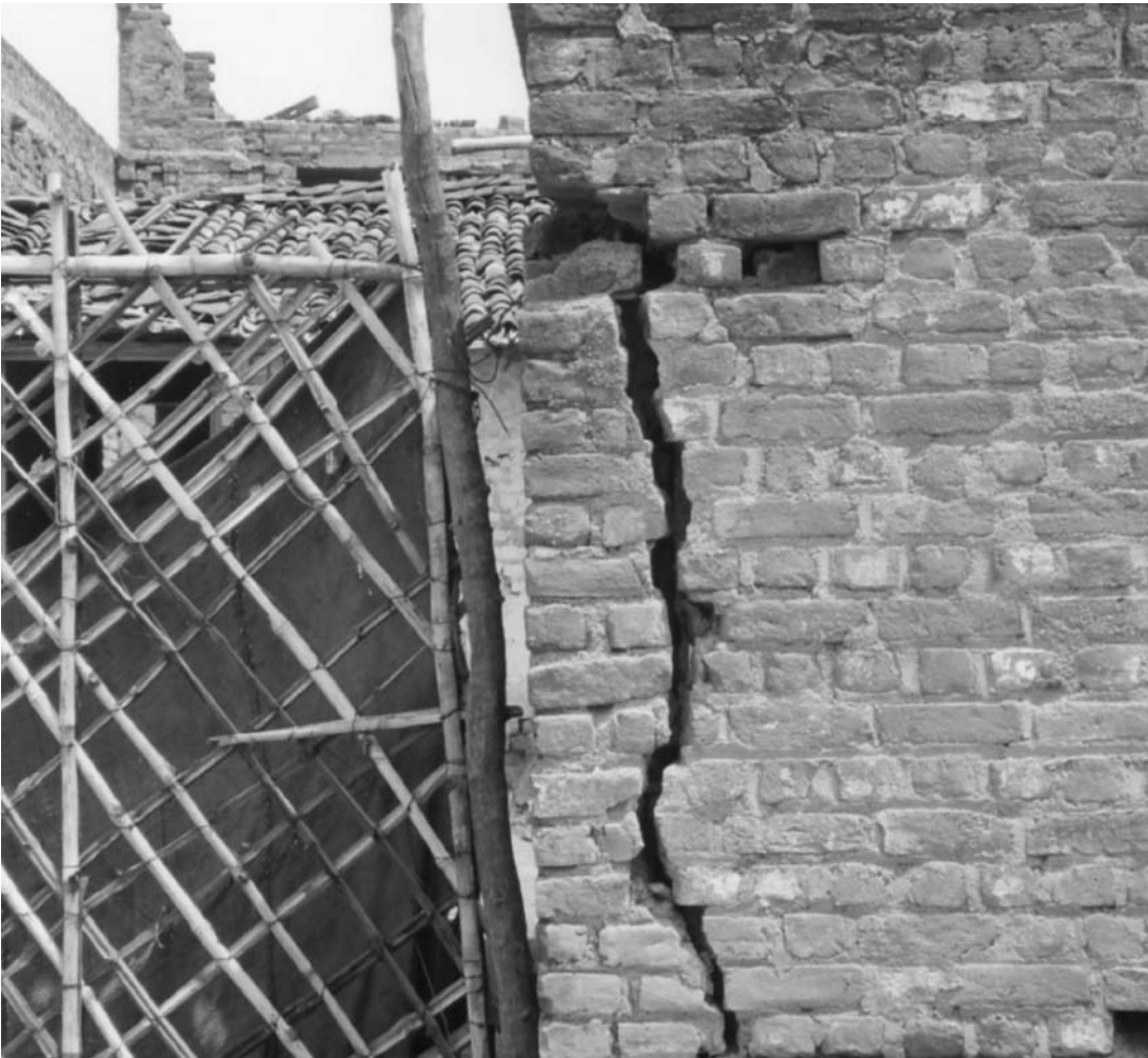
Bad brick wall construction resulting into corner collapse / damage
