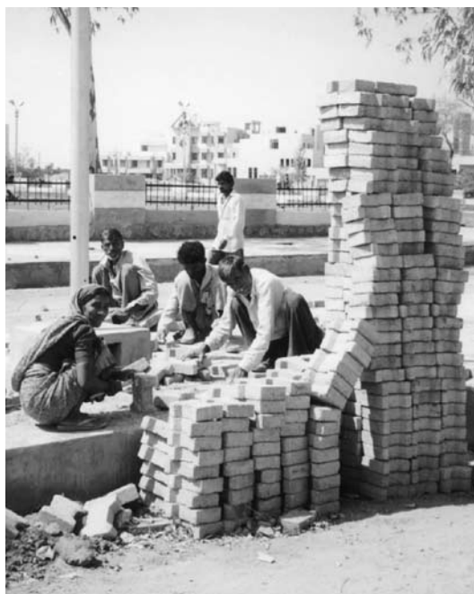
Pavement blocks dangerously piled up, workers at increased risk of accident
