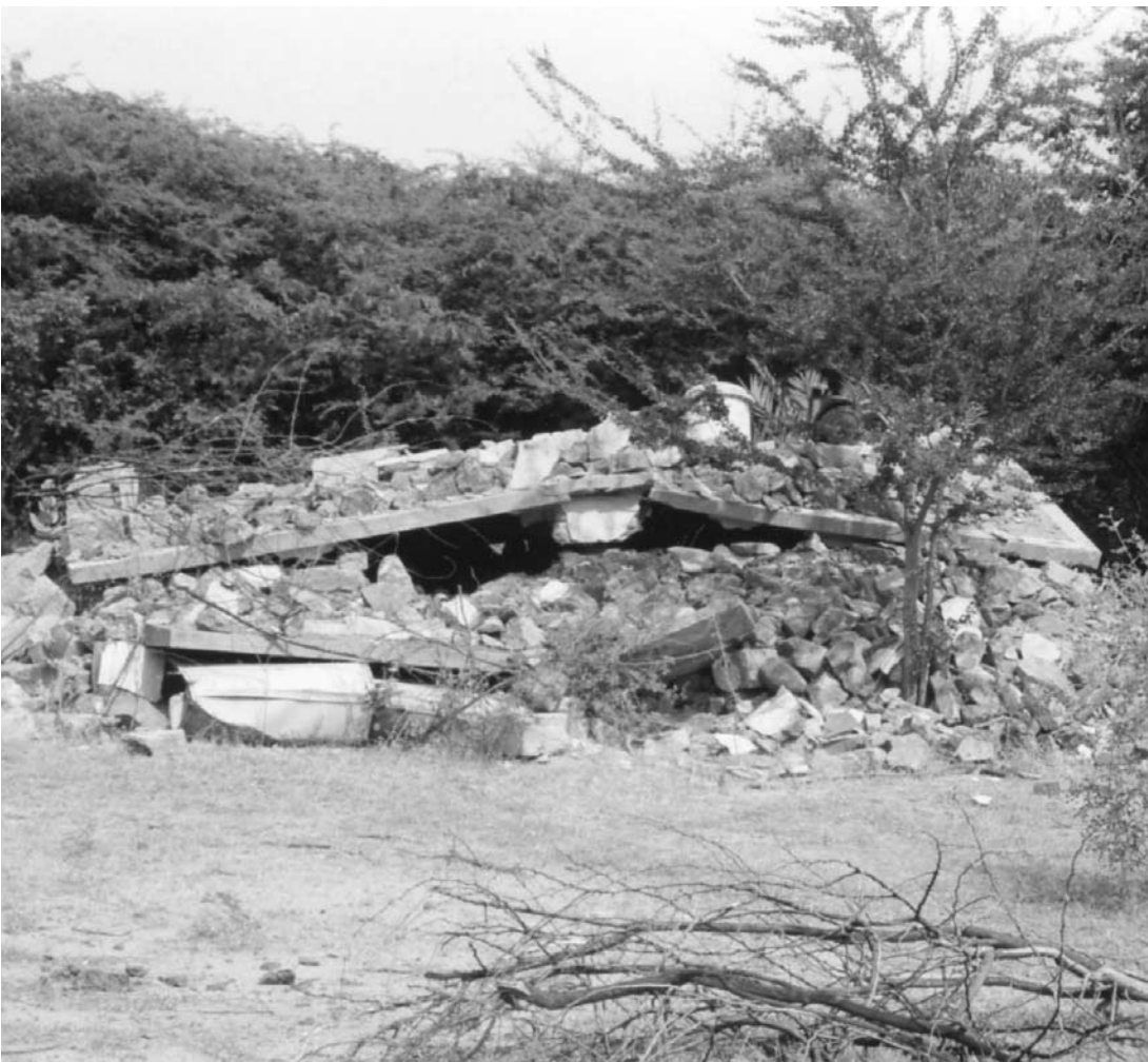
Remains of one story building collapsed during earthquake
