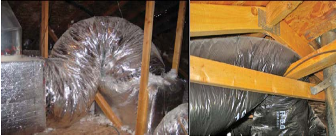
Figure 2. Examples of constricted ducts (Photo credit: R. Chitwood, reprinted with permission).
